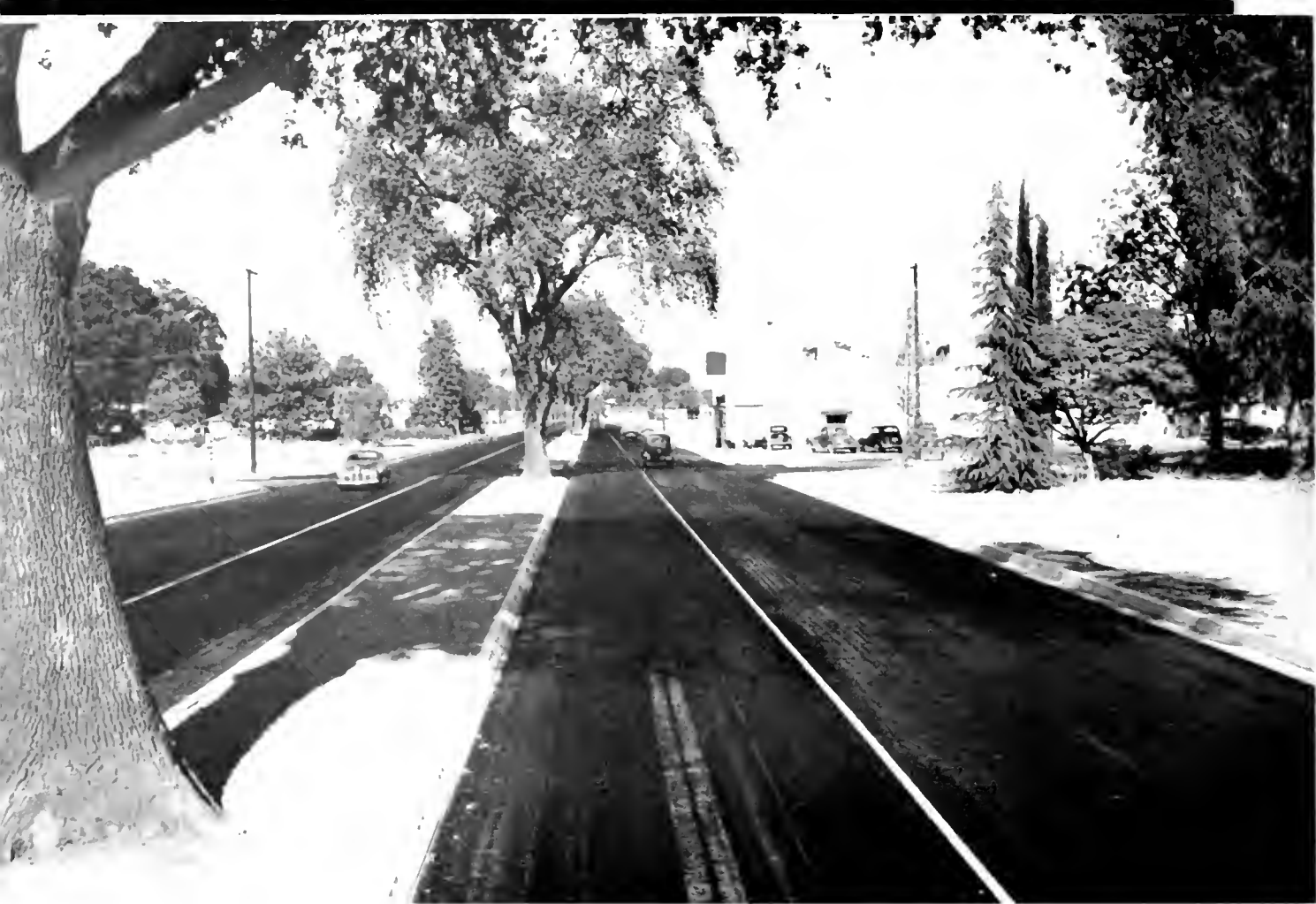
Many large, beautiful trees were saved in construction of the division strip on new 4-lane highway section through Visalia
